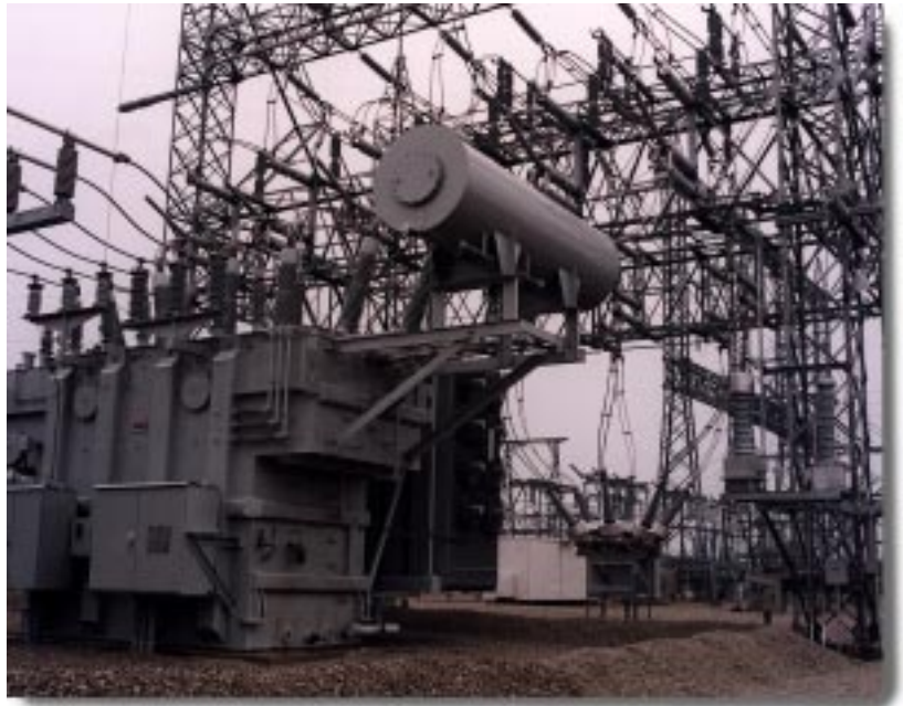
UPFC series transformer
